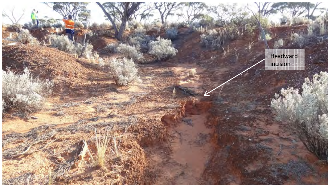
Figure 14. Headward incision in the channel of an existing watercourse in the southern corridor
